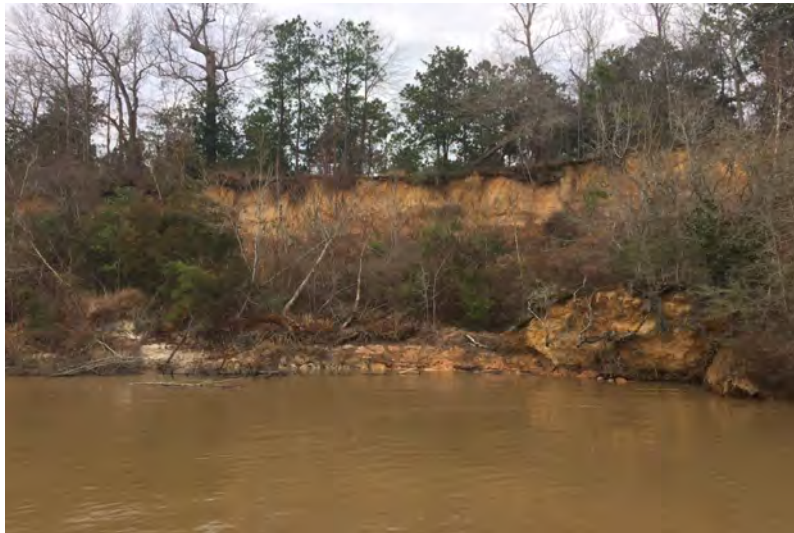
Photo 4: Flooding Adjacent to Barry Ash Pond (Jan. 3, 2016)
