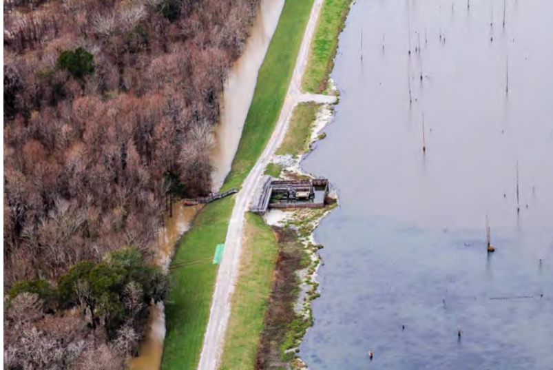
Photo 3: Evidence of River Bank Erosion (Feb. 9, 2017)
